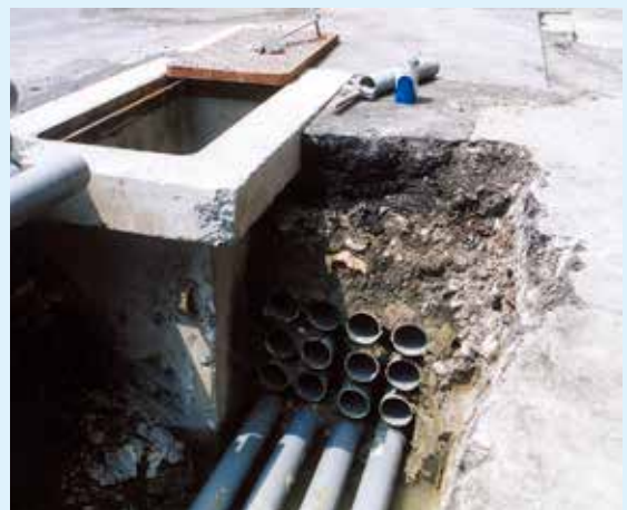
固網通訊工程 Cable net-work communication engineering
